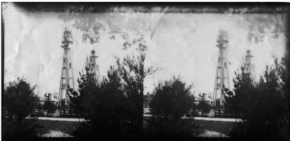
Fig 41. 'Stereoscopic glass slide of old wooden lighthouse and present lighthouse (1883) in process of construction'
